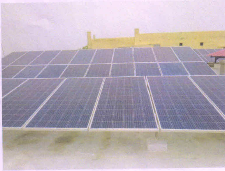
Fig-Solar Energy Generation System
